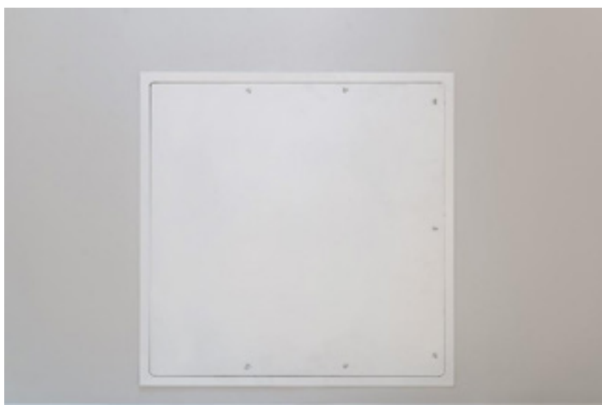
Ceiling-mounted ERV access
