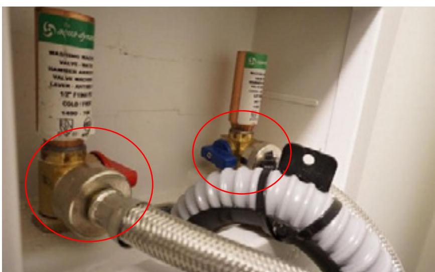
Washer water shut off valves. One valve will always be facing away from you within the cavity, so be mindful to switch both off in case of a leak.
