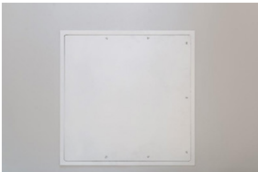
Ceiling-mounted ERV access
