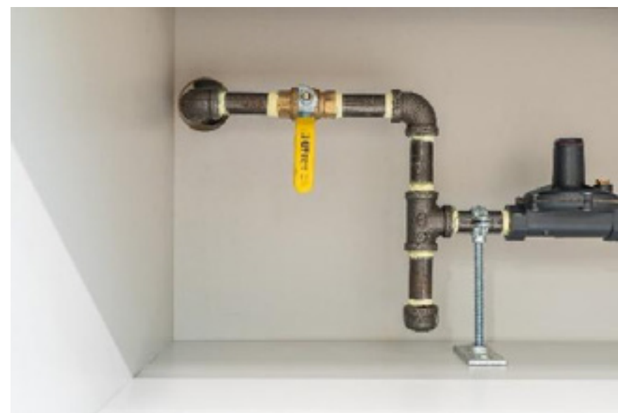
Gas shut off in the “off” position.
