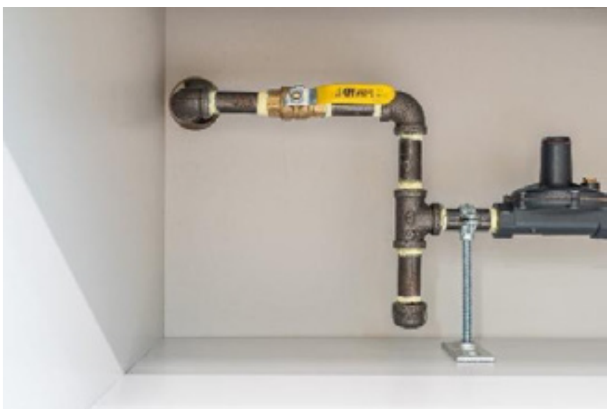
Gas shut off in the “on” position.
