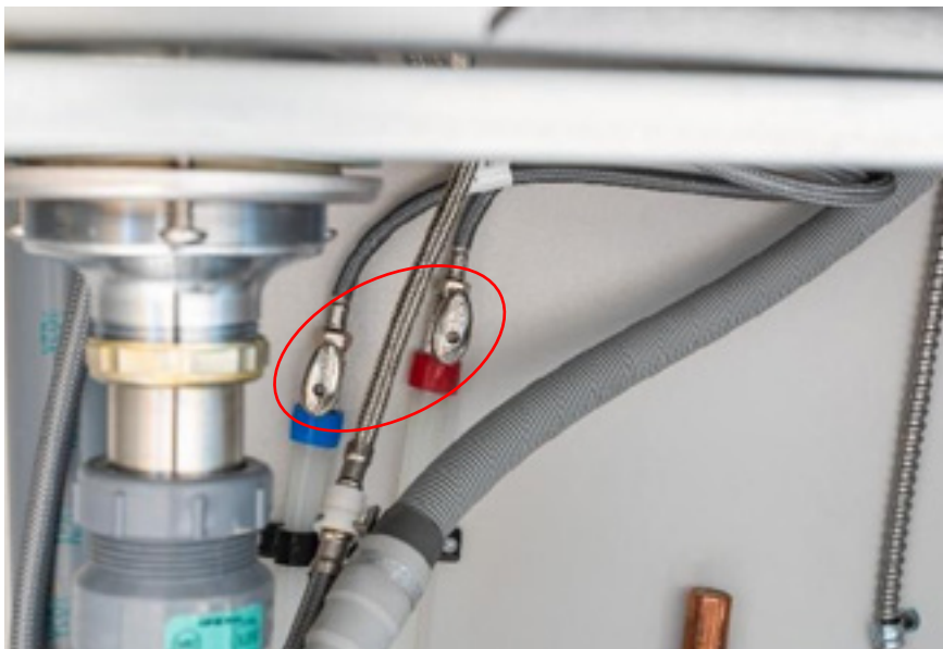
Faucet shut offs below kitchen sink.
