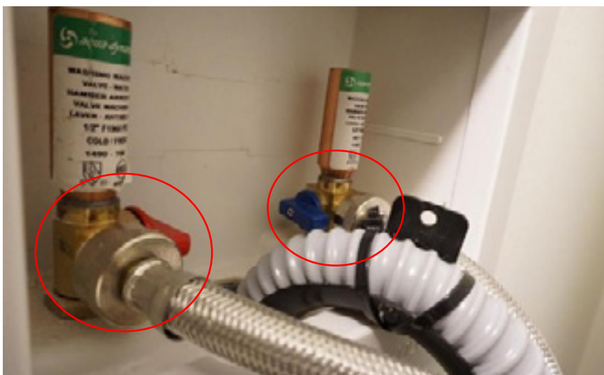
Washer water shut off valves. One valve will always be facing away from you within the cavity, so be mindful to switch both off in case of a leak.
