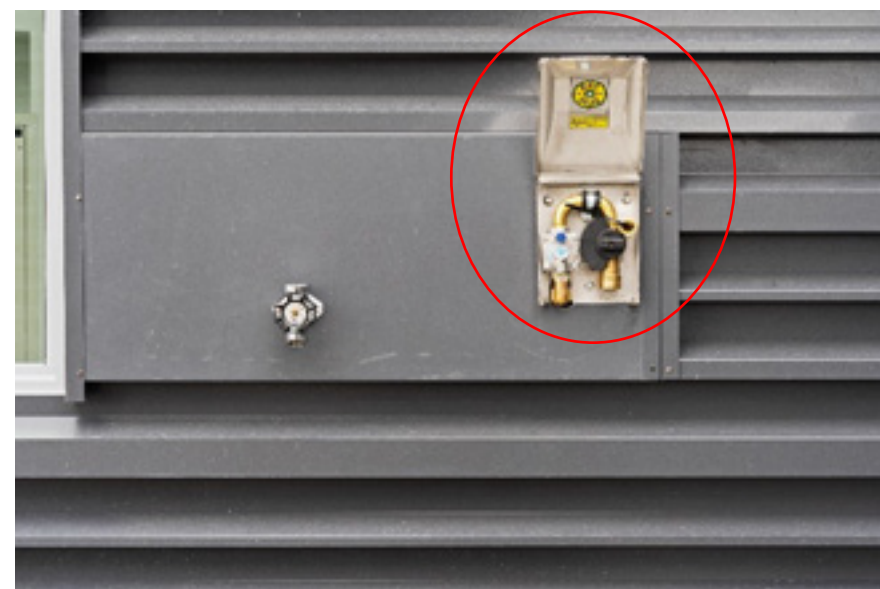
Gas shut off with cover opened.
