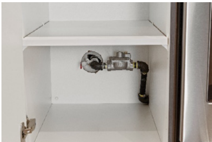
Gas shut off location for the cooktop.
