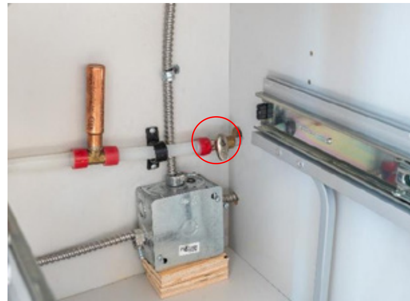
Be mindful that your dishwasher water shut off may be behind the rolling waste bins.
