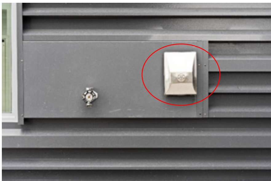
Gas shut off with cover closed.
