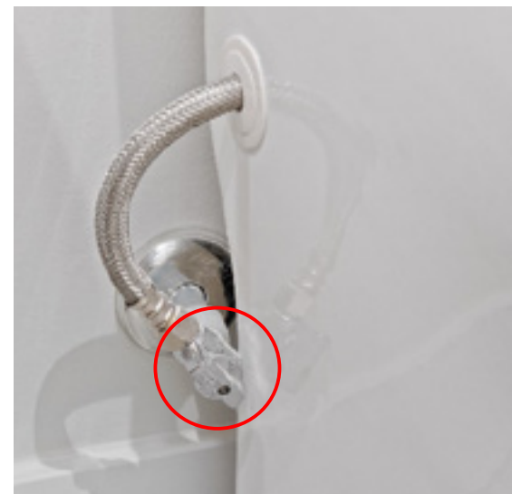
Toilet shut off behind the toilet.
