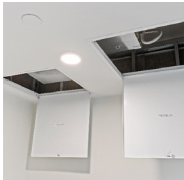
The heat pump with covers open
