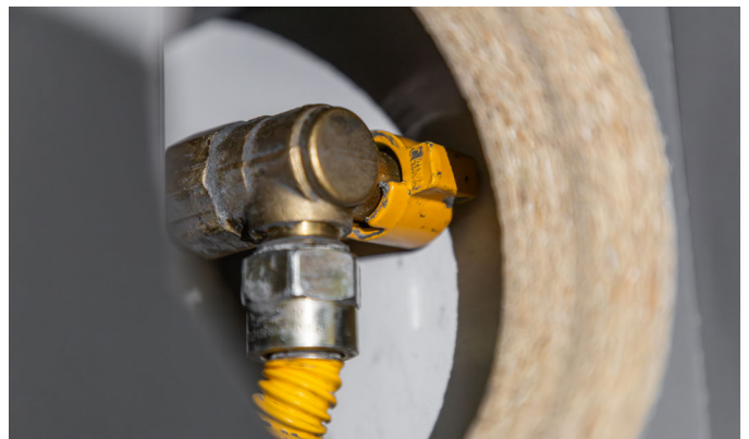
To shut off the gas, turn the valve to the off position
