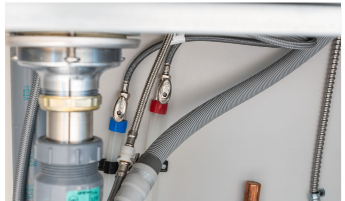
Faucet shut offs below kitchen sink.
