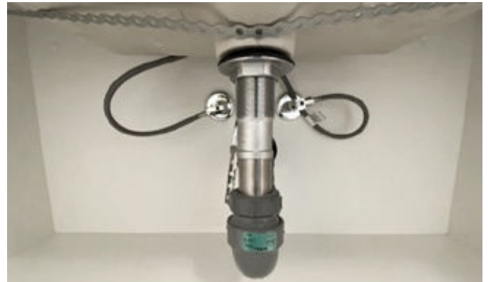
Bathroom faucet shut offs below bathroom sink.
