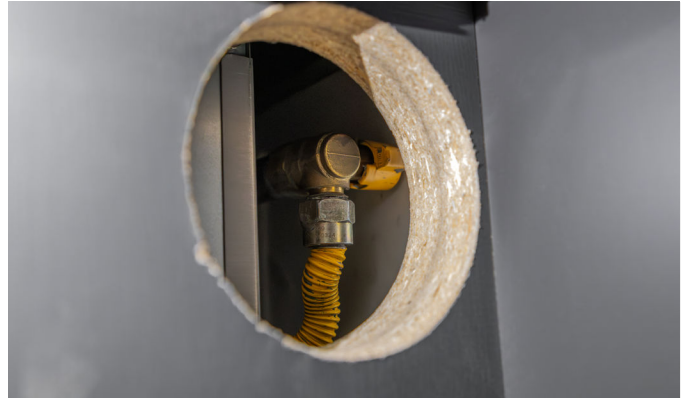
Gas shut off valve
