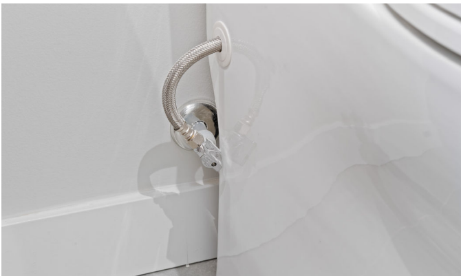
Toilet shut off behind the toilet.
